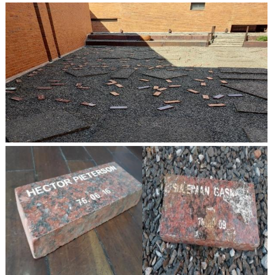
Image 2 : Court yard condition & granite slab
