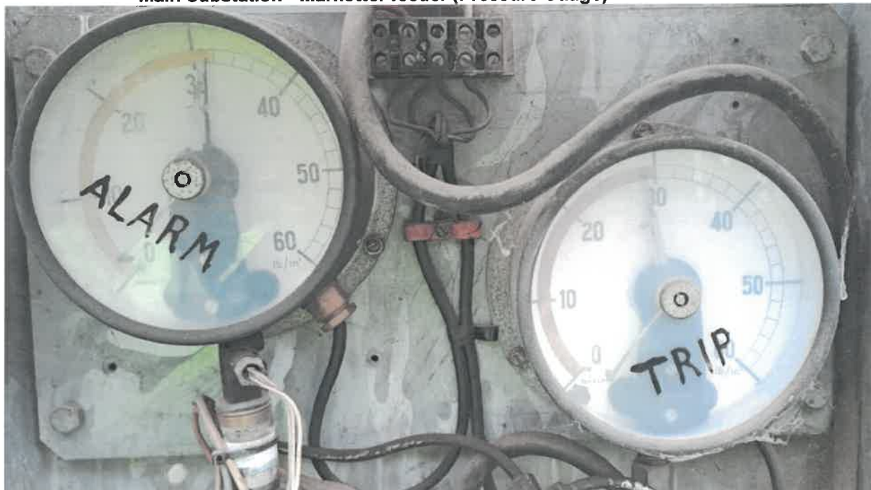
Main Substation - Markotter feeder (Pressure Gauge)
