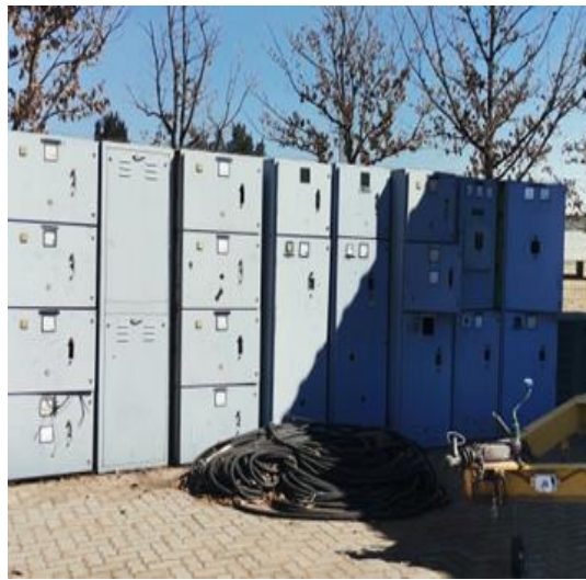
10 x Electric panels
