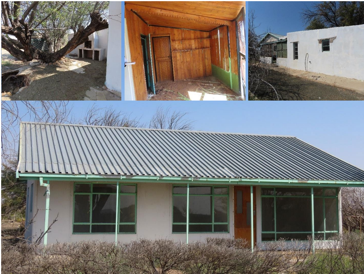
Figure 3: House No.2 – Made of a combination of asbestos cladding and roof sheeting, wood and brickwork. (asbestos to be removed & entire building to be demolished)
