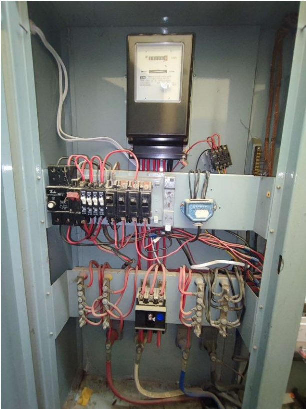
Existing MDB – Municipal Meter
