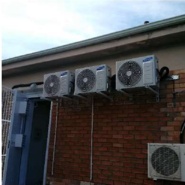
Figure 1: 3 x 18 000 BTU air conditioners installed at BBI George
