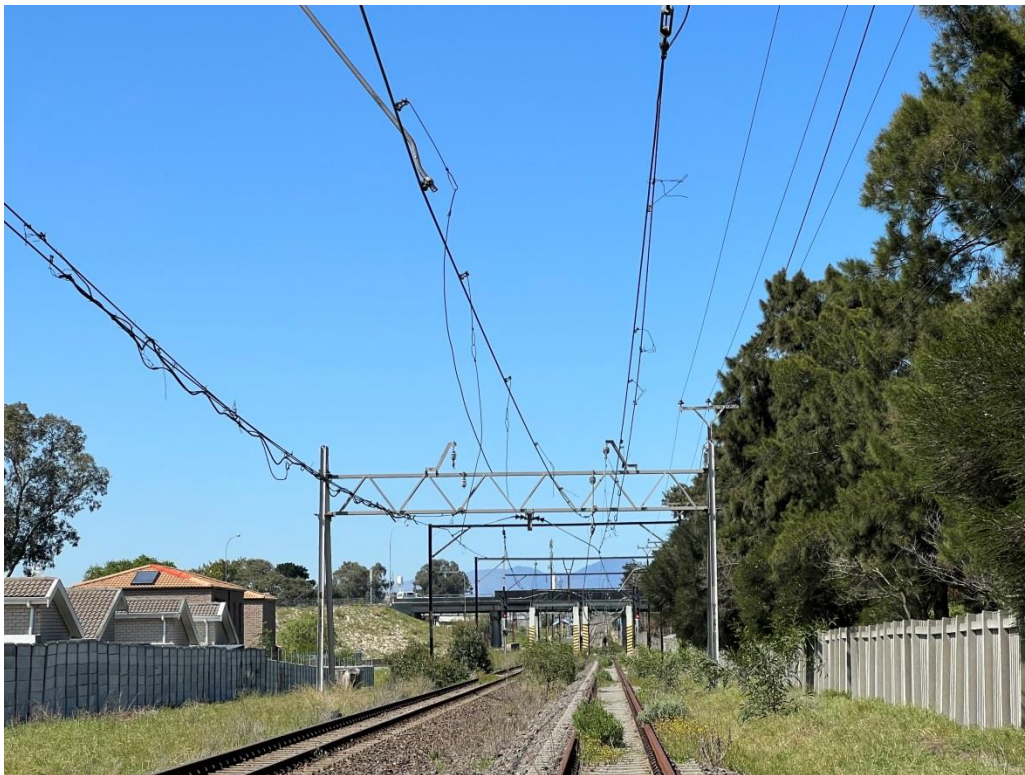
Figure 2 Damaged Ohte Lines
