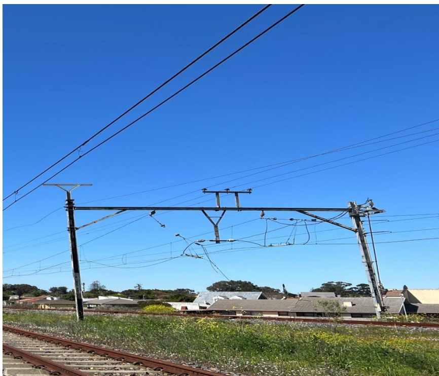
Figure 4: vandalised and Stolen OHTE
