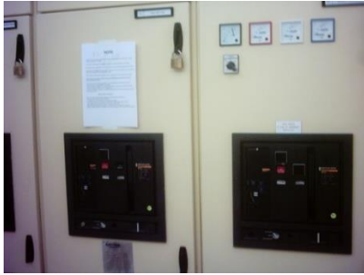
400V Incomer CB's on MCC board view
