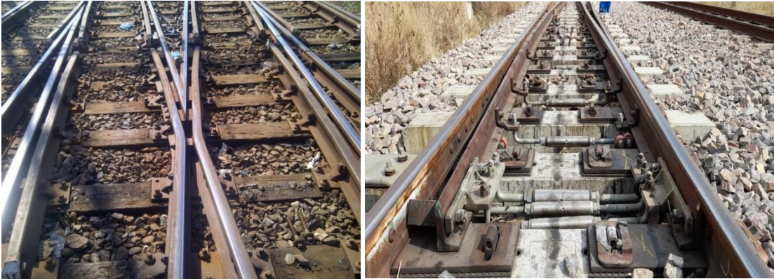
Figure 1: Wooden sleepers and stolen railway fastening clips on a turnout crossing.
