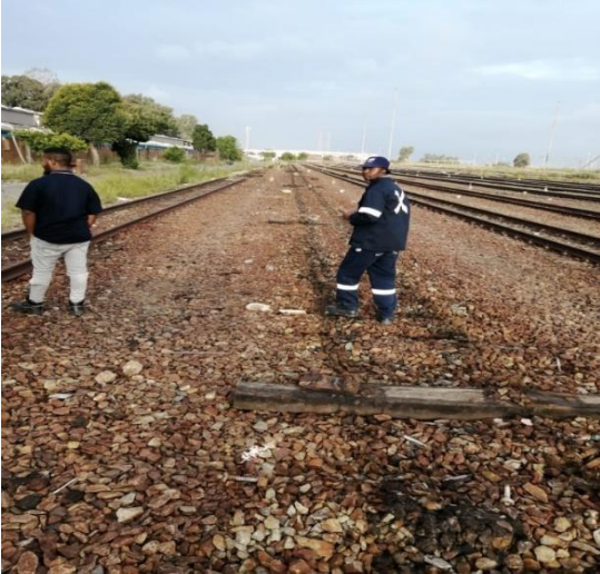
Fig 2.1: Missing sleepers and vandalised track
