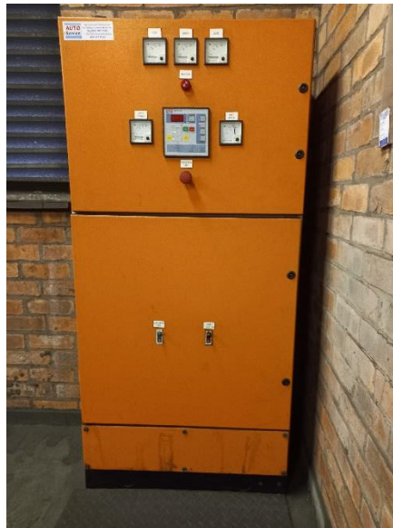
Figure 1: Existing Transtel Control Panel.
