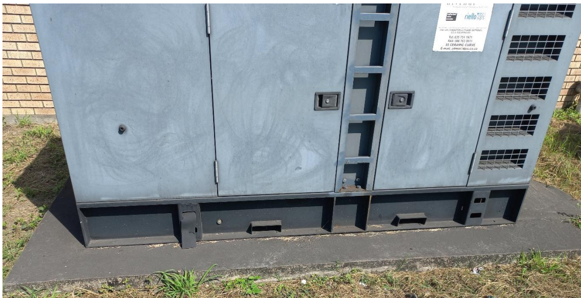
Figure 2: Similar Concrete Plinth for Berthing Generator.
