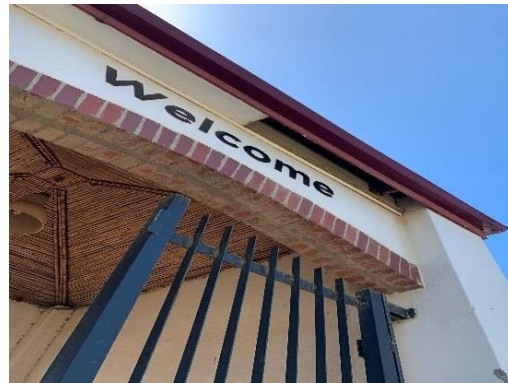
FIGURE 1.4: Replace missing eaves ceilings
