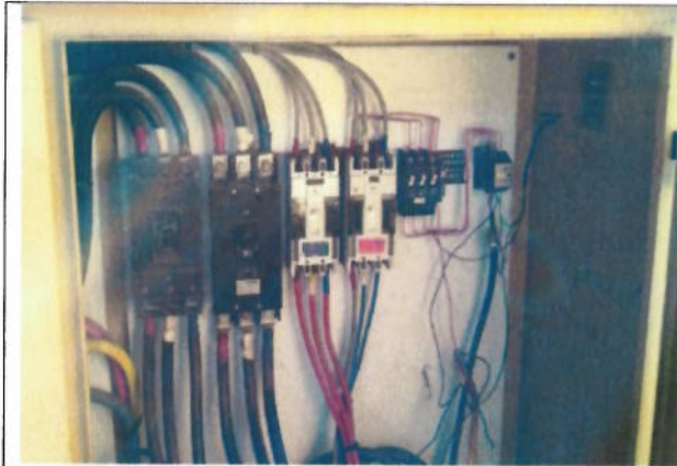
Picture 1 Distribution box
