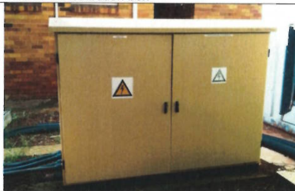
Picture 3 Distribution box
