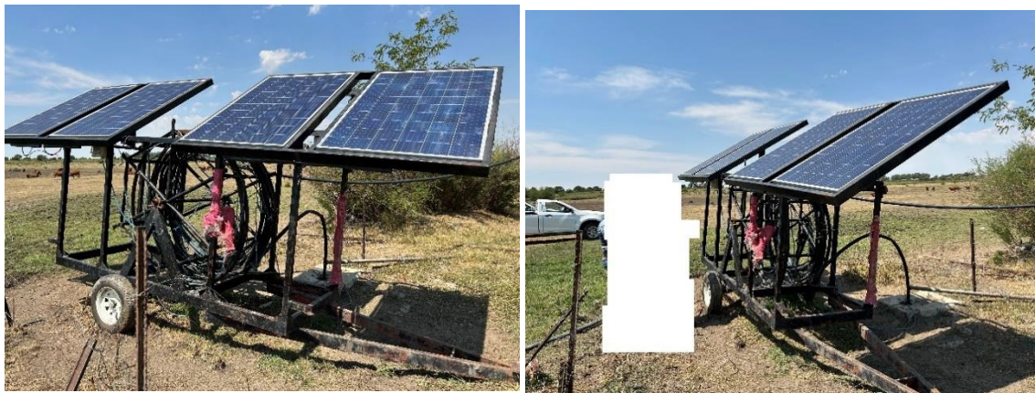
Fig.1: Mobile solar power system with 4 panels, single axle, submersible pump, and water pipe.
