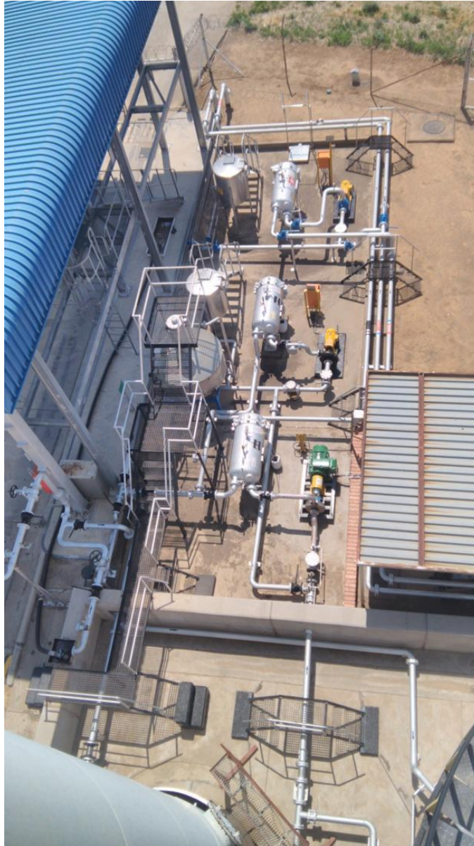
BFA – Filtration Station
