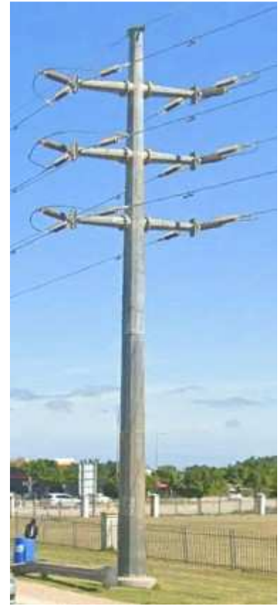
Photo 3. Typical Strain Structure (Single Pole)
