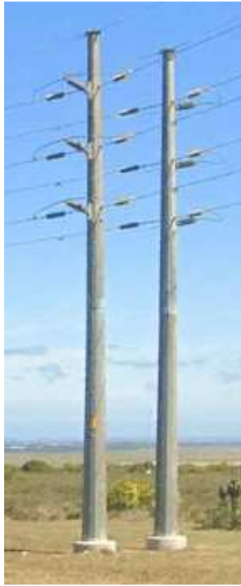
Photo 2. Typical Strain Structure (Double Pole)
