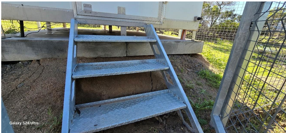
Figure 2: CTHIS FB Subbase structure washing away from beneath the concrete plinth
