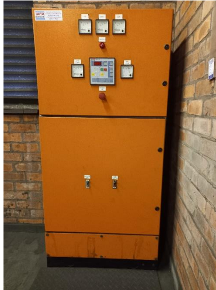
Figure 1: Existing Transtel Control Panel.
