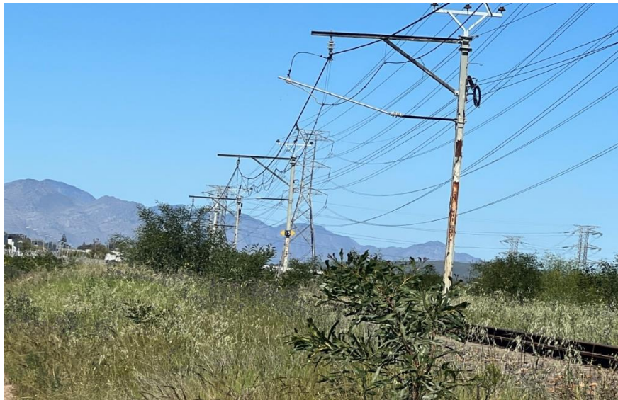
Figure 4: vandalised and Stolen OHE
