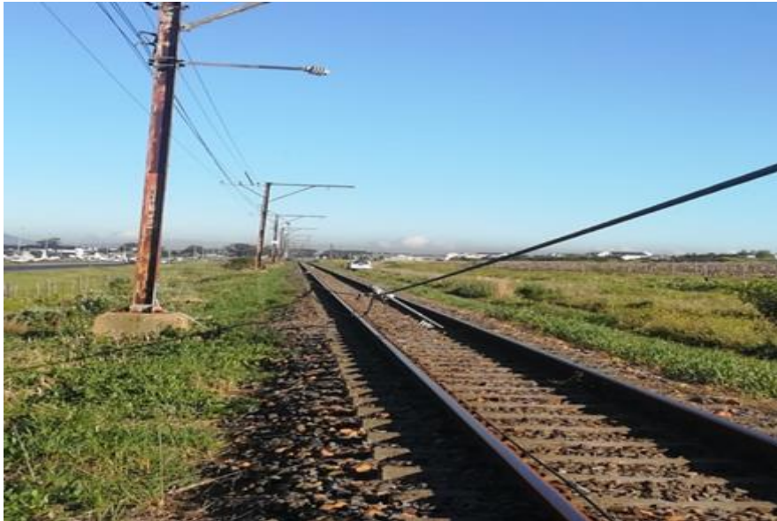
Figure 2 Damaged OHTE Lines
