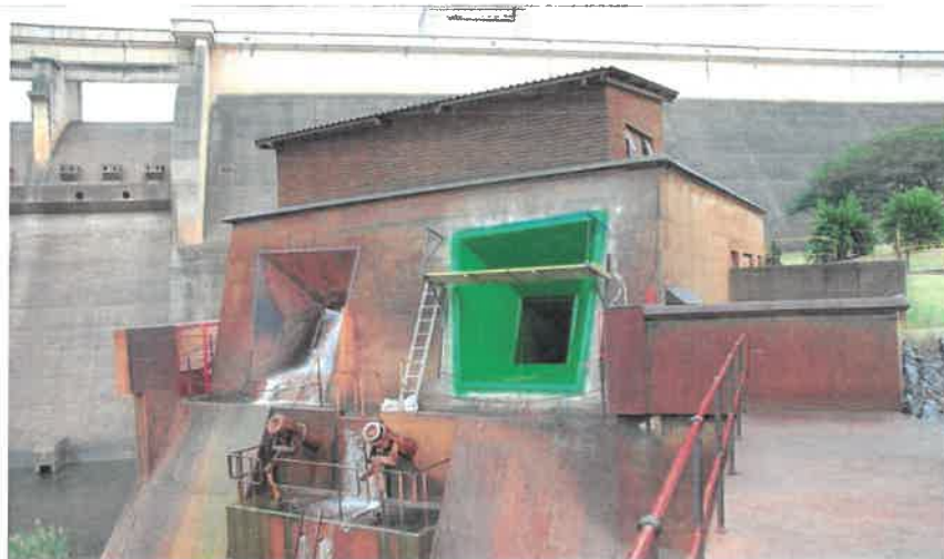
Outlet control room with Jetflow valves and Sleeve valves.
