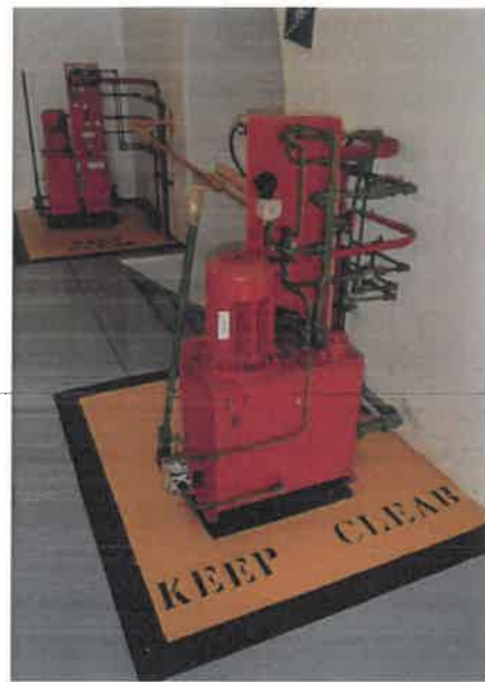
Sleeve valve power packs
