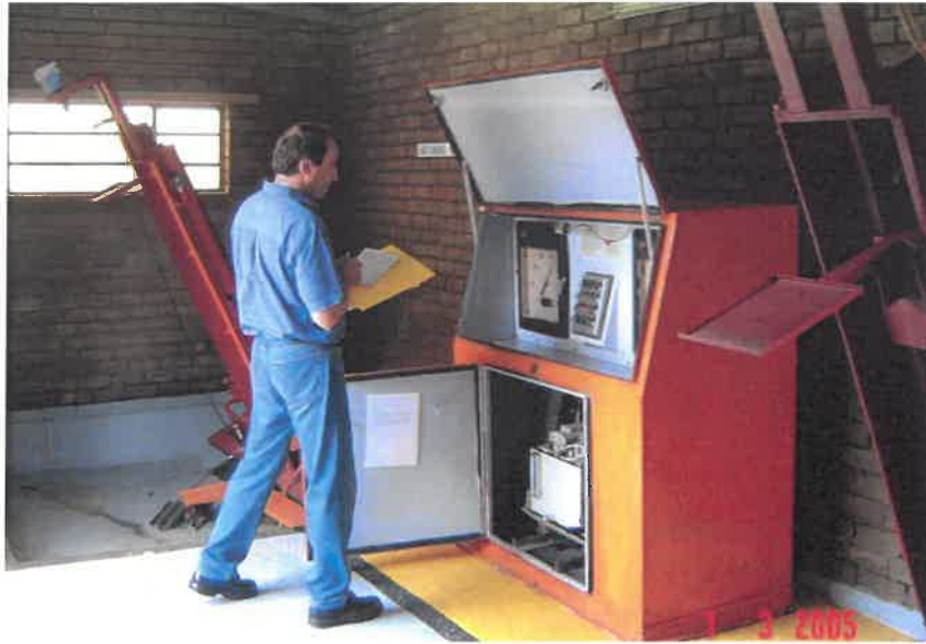
Jetflow valve power pack and hydraulic cylinders
