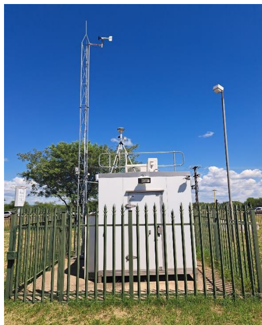
Example of an Air Quality Monitoring Station
