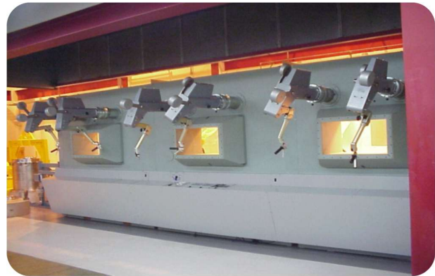
Figure 5: Example of hot cells at a research reactor facility
