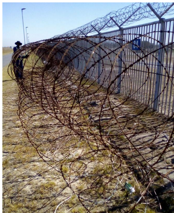
Figure 1 - Razor coil on the inside of the fence that must be removed prior to cutting.
