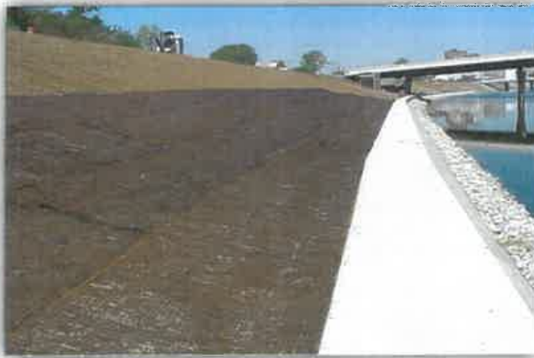
Figure 2 Geo-fabric installed and pegged down on a slope to retard soil erosion. Vegetation may grow through the blanket over time.
