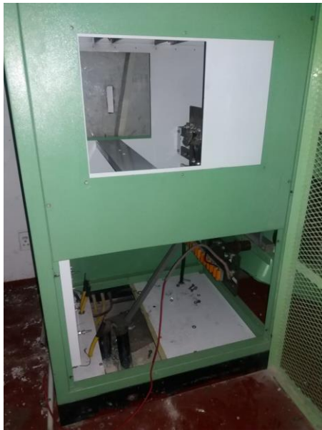
Figure 3: Chris Hani 3KV Positive Isolator
