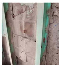
Condition of front wall plates
