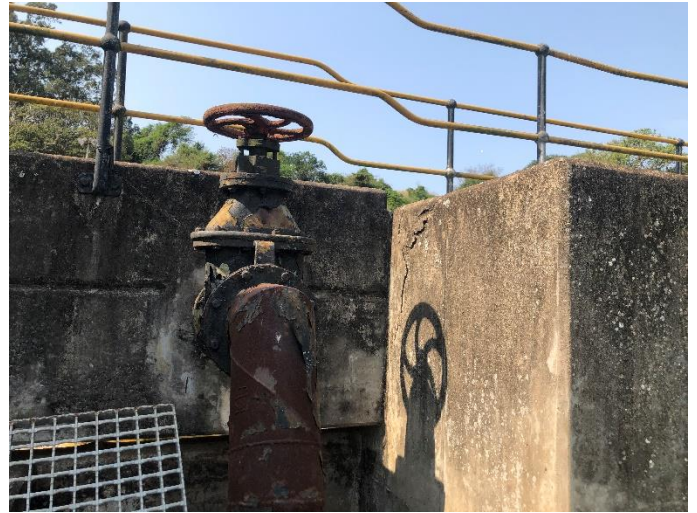
Screw Pump Room Photo 15-Beam Spalling
