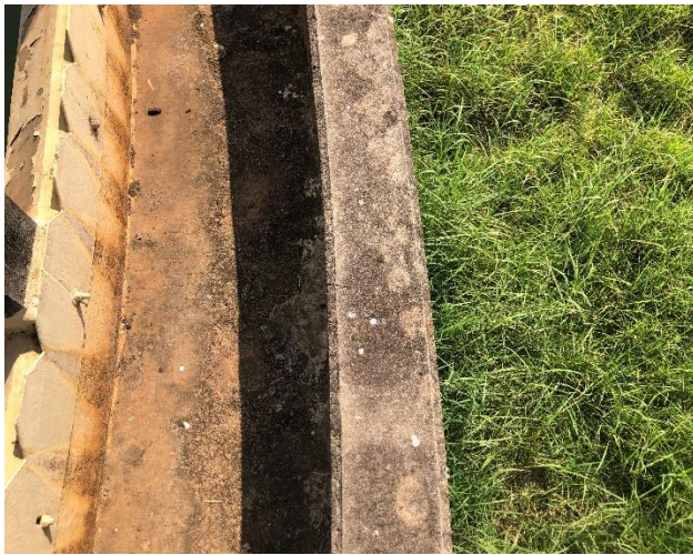
Clarifier (2) Photo 07-Outer wall cracks (0.2-0.3mm)
