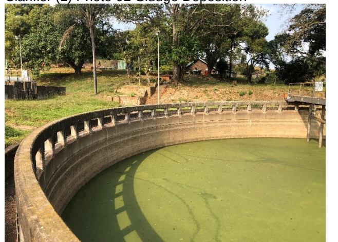
Clarifier (1) Photo 03-Water in Clarifier.
