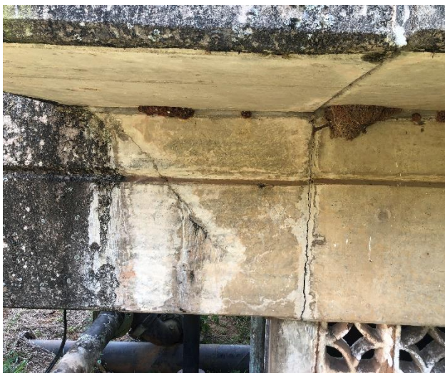
Screw Pump Room Photo 14-Diagonal crack on beam
