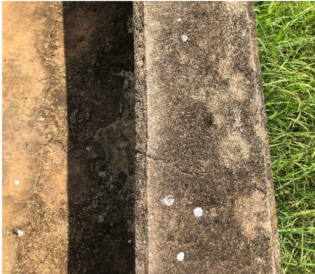
Clarifier (2) Photo 09-Detail outer wall cracks (0.2-0.3mm)
