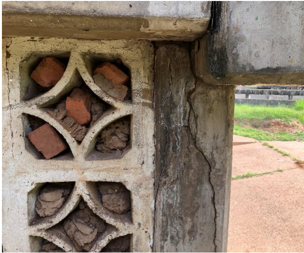
Screw Pump Room Photo 13-Failed expansion Joint and column spalling
