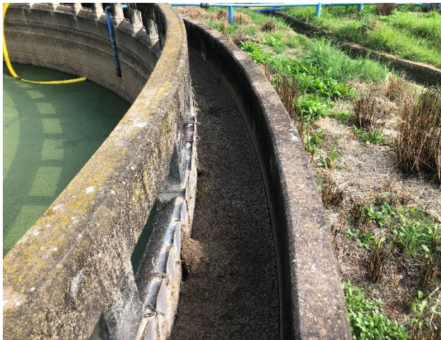
Clarifier (1) Photo 01-Sludge Deposition
