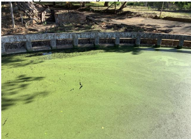
Clarifier (1) Photo 01-Shows Tilt
