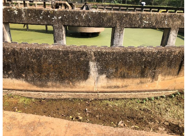
Clarifier (1) Photo 06-Outer wall cracks (0.2-0.3mm)
