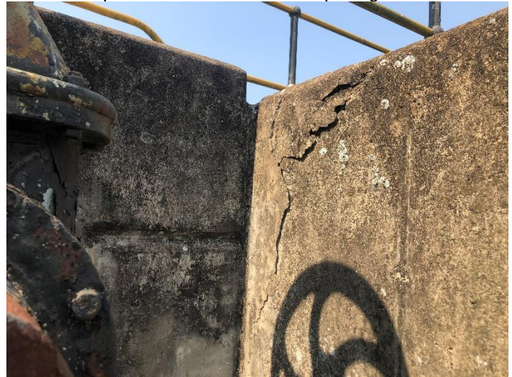
Screw Pump Room Photo 16-Deatil Beam spalling
