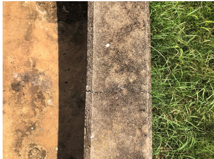
Clarifier (2) Photo 08-Outer wall cracks (0.2-0.3mm)
