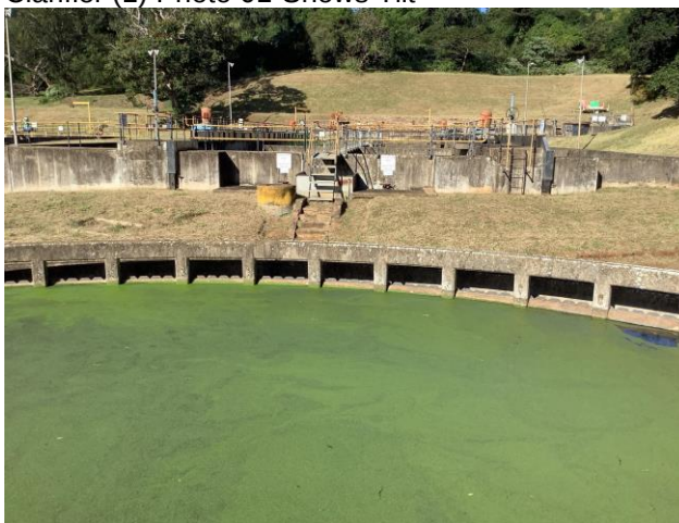
Clarifier (1) Photo 01-Shows Tilt
