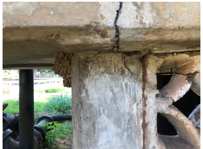
Screw Pump Room Photo 12-Failed expansion Joint and column spalling
