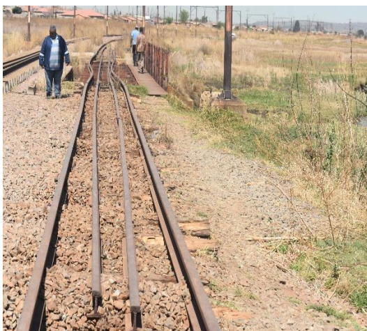
Fig 2.3: Stolen wooden sleepers at Residensia
