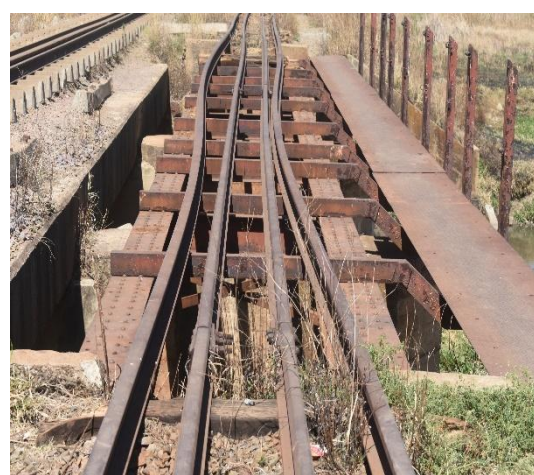
Fig 2.4: Stolen sleepers at Stretford – Residensia bridge
