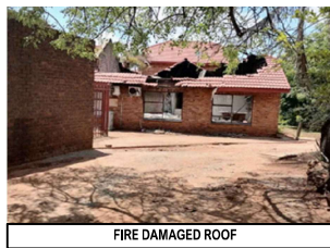
FIRE DAMAGED ROOF
