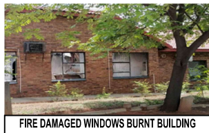
FIRE DAMAGED WINDOWS BURNT BUILDING
