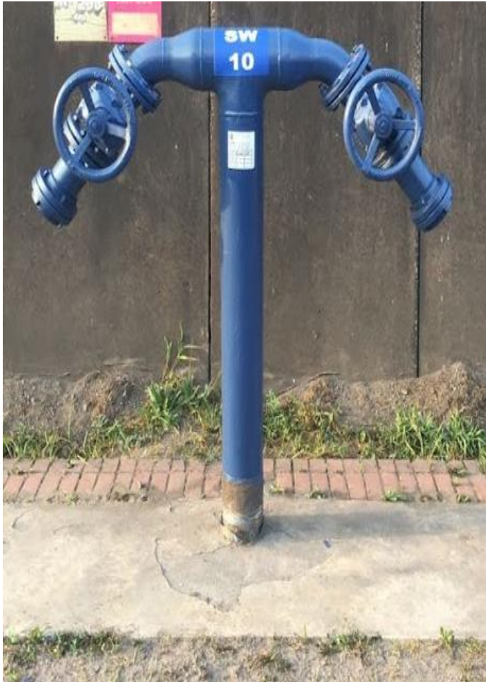
Two Spouts Hydrants
