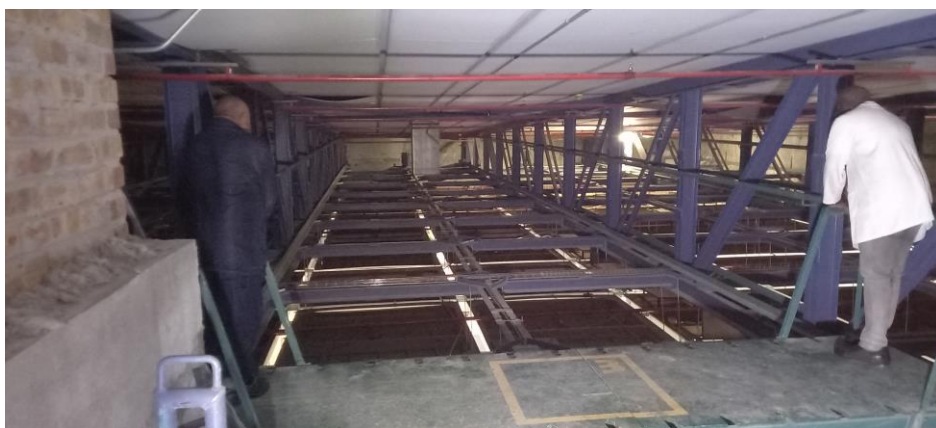
Figure 2 Trolleys that need to operate on tracks to access winches.
