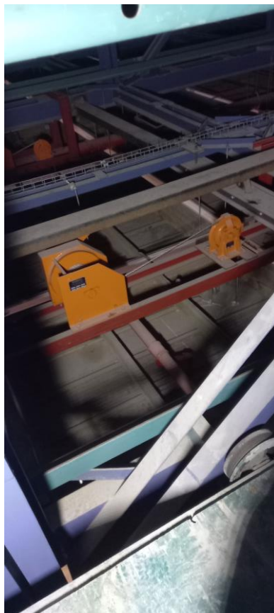
Figure 5 Winches to be serviced that suspends whales with steel cable.
