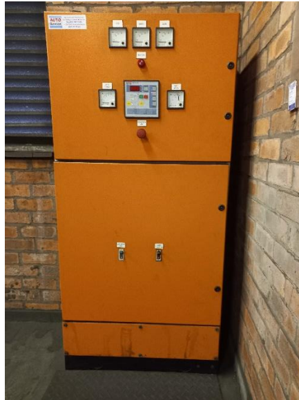
Figure 1: Existing Transtel Control Panel.
