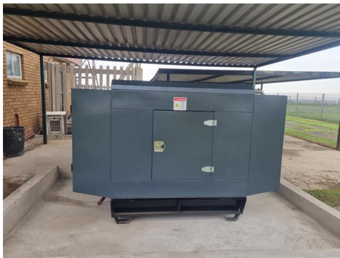
Figure 1: Ermelo Diesel generator
