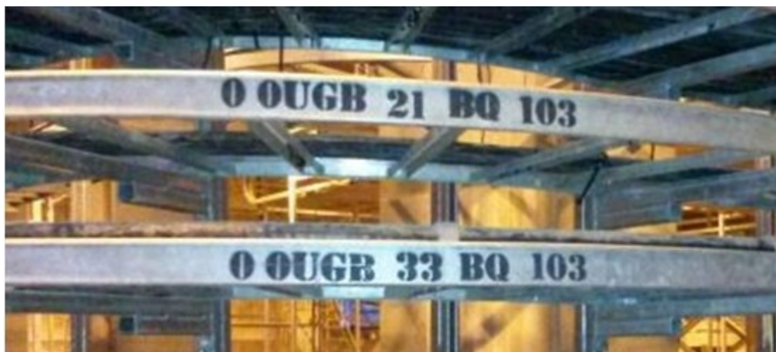
Figure 31: Cable rack label
