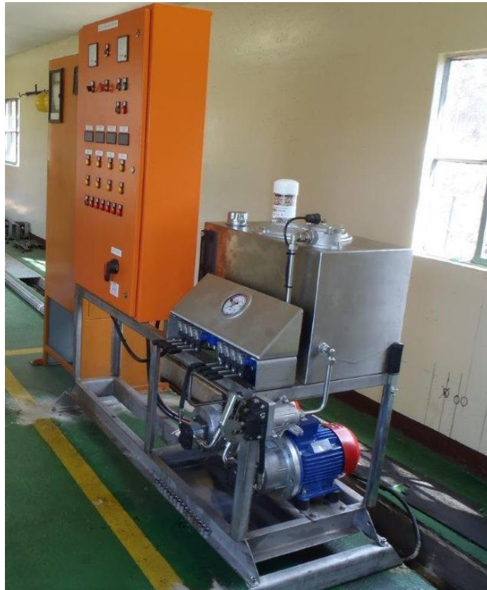
Pongolapoort dam: Canal outlet Hydraulic power pack
