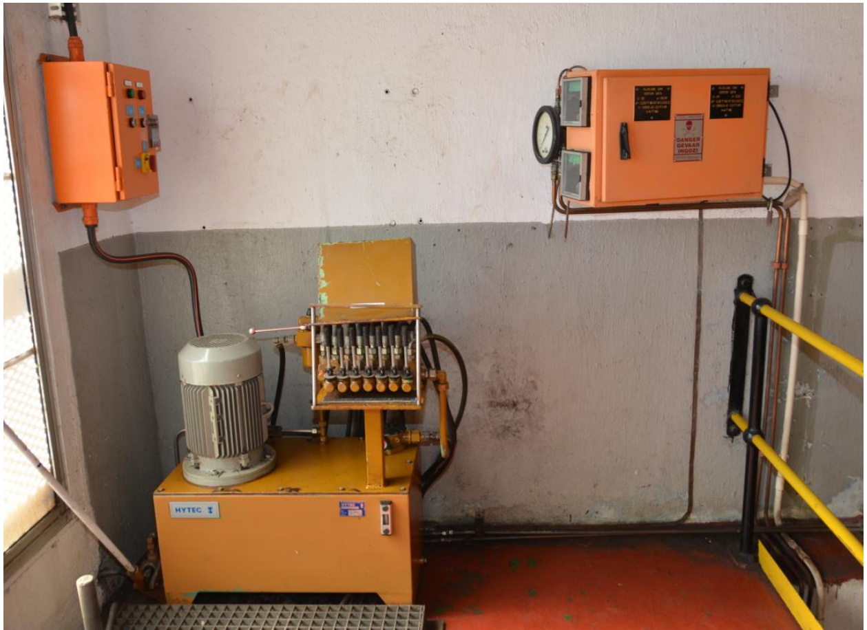
Hluhluwe dam: Outlet control room: Hydraulic power pack in.
