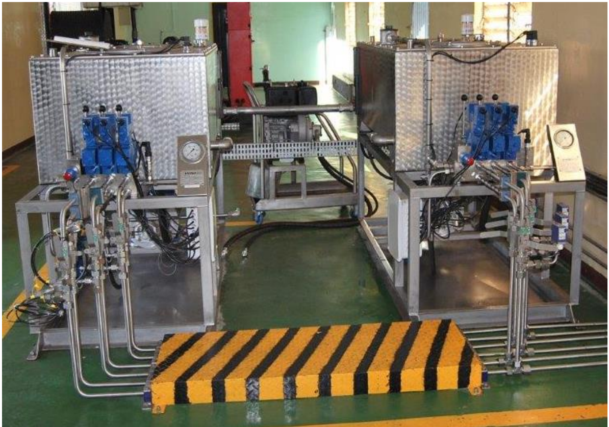
Pongolapoort dam: radial gate hydraulic power pack
