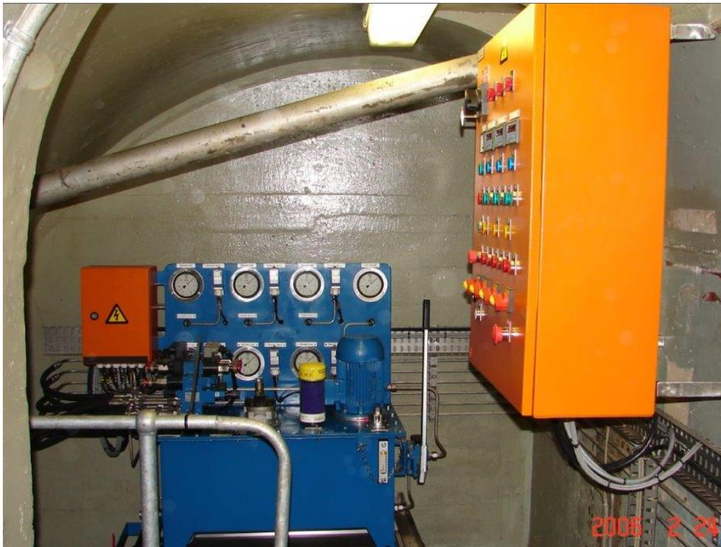
Ntshingwayo dam: River outlet: Hydraulic power pack
