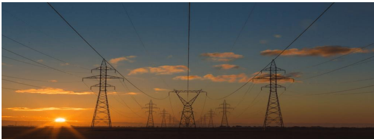
Electricity Power Lines
