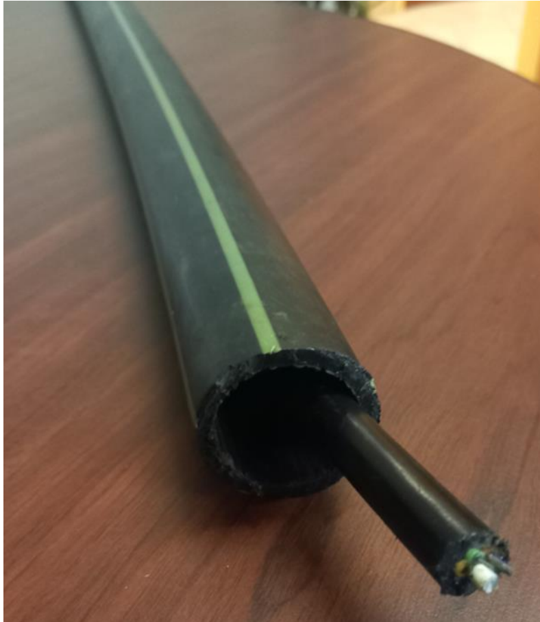
Figure A1: Current “conducted” 48 Core single-mode fibre cable installation.
