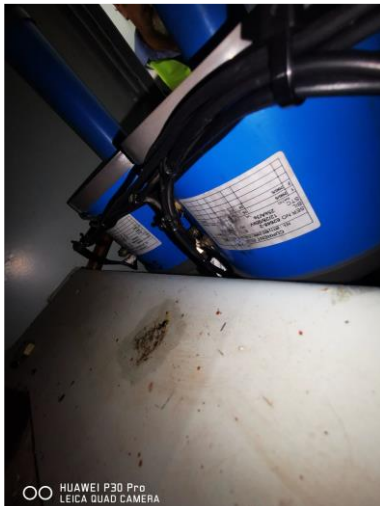
Figure 1 – 11kV Incomer CT
