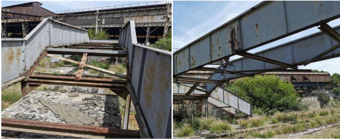
Figure 2: Structural Steel Corrosion
