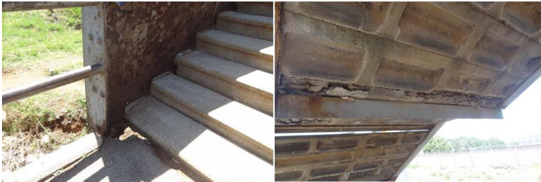
Figure 3: Precast staircase defects
