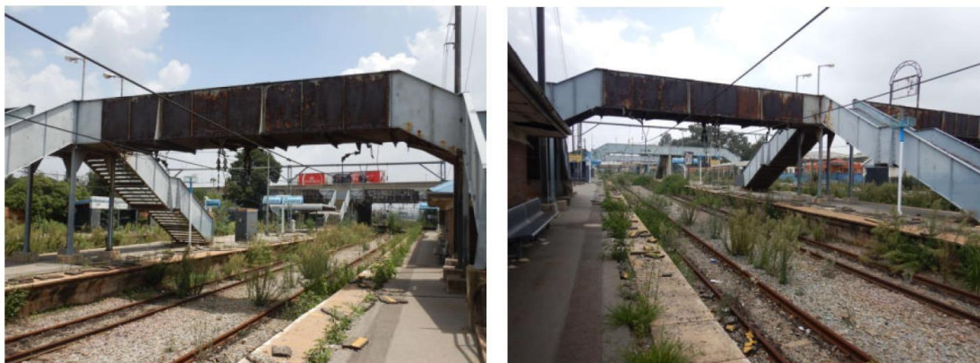
Figure 1: Parapet Steel Corrosion
