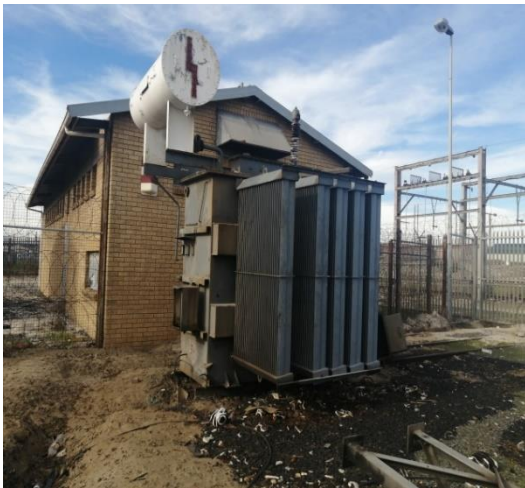
Figure 1: Nolongile 3kV DC Sub Traction Transformer
