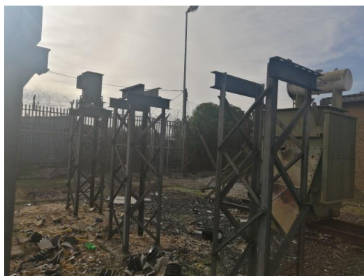
Figure 5: Nolongile 11kV Outdoor Yard
