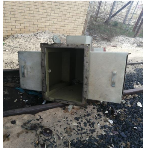
Figure 2: Nolongile 3kV DC Sub Aux Transformer
