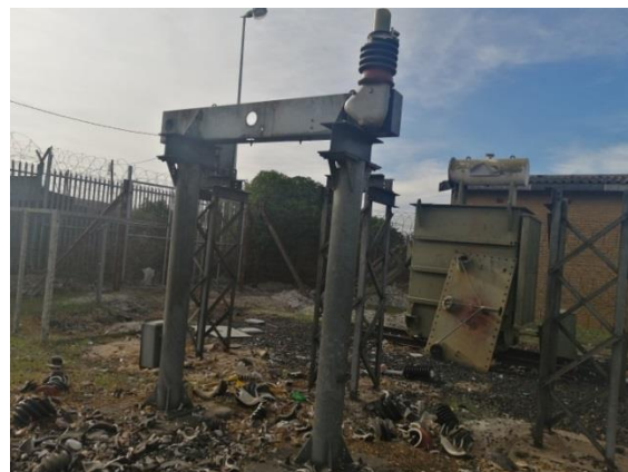
Figure 4: Nolongile 11kV Outdoor Yard (Signal unit)
