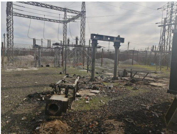
Figure 3: Nolongile 11kV Outdoor Yard (Signal Unit)
