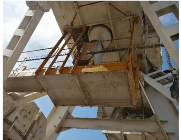
Figure 4: Current condition of the Cranes Undercarriage.
