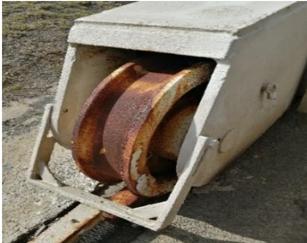
Figure 5: Current condition of the Cranes wheels
