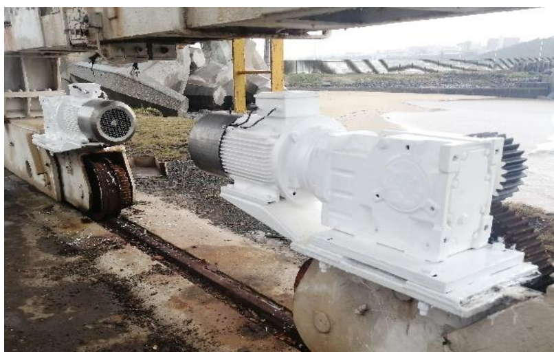
Figure 3: Current condition of the Drive Motors
