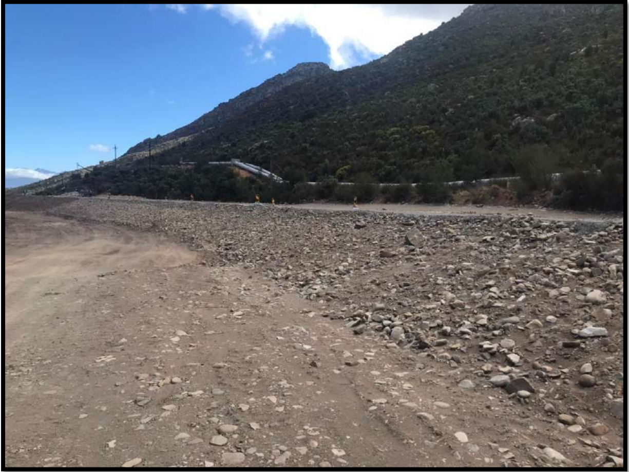
FIGURE 13: BARE EMBANKMENT ALONG STETTYNS ROAD.
