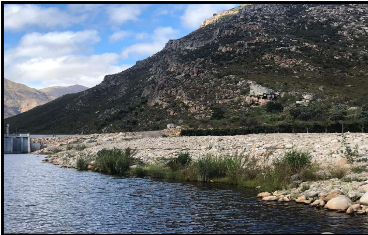
FIGURE 16 BARE EMBANKMENT; DOWNSTREAM OF WEIR; LEFT EMBANKMENT.
