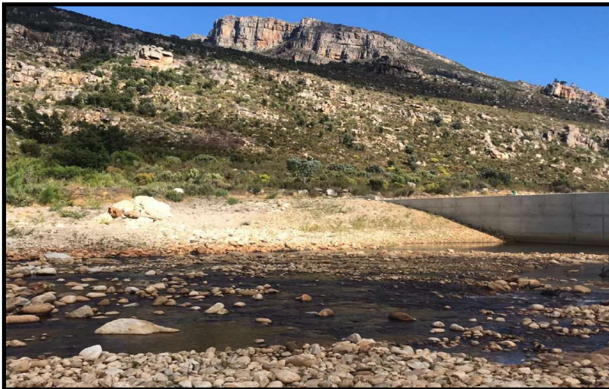
FIGURE 14: BARE EMBANKMENT; UPSTREAM OF WEIR; LEFT EMBANKMENT.
