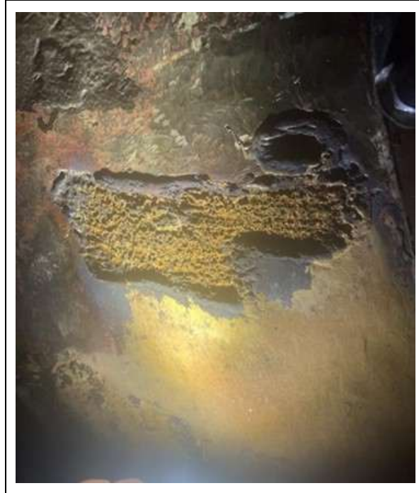
Figure 1: Spiral casing typical liner damage
