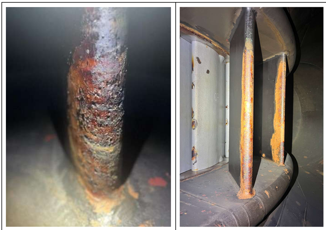
Figure 2: Example of typical damage on vertical stay vane
