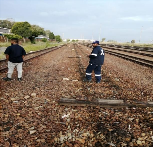
Fig 2.1: Missing sleepers and vandalised track
