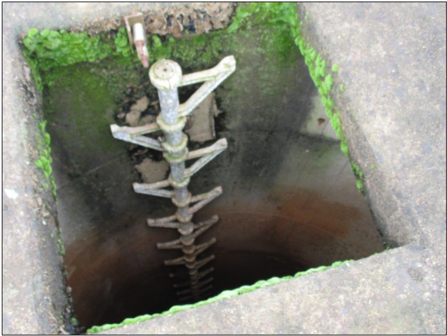
Figure 8: Current ladder inside tower
