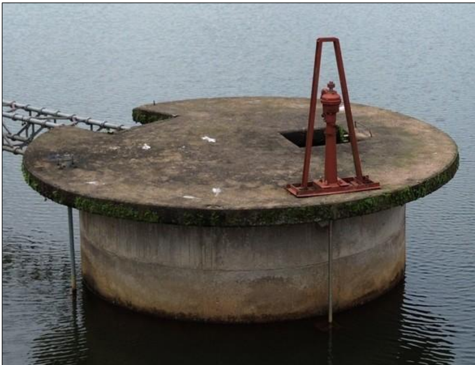
Figure 9: Intake tower sluice gate controls
