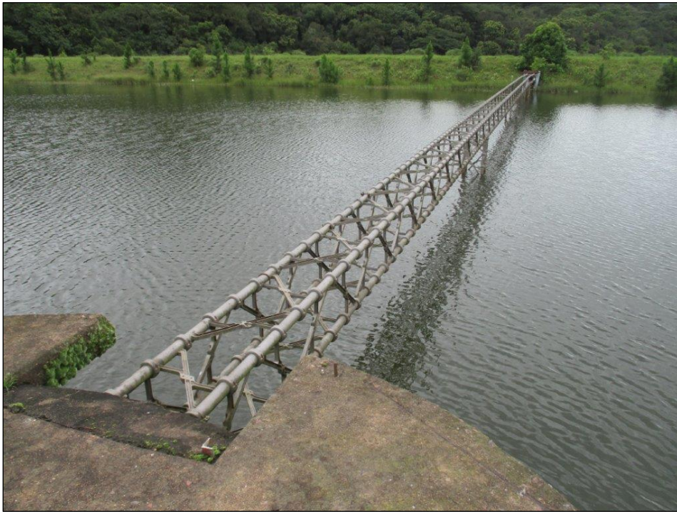
Figure 11: Remains of old walkway
