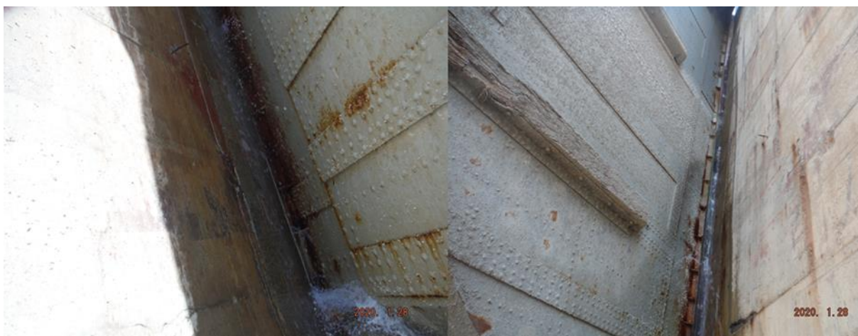
Figure 8: Leaks at Dock Gate Grooves
