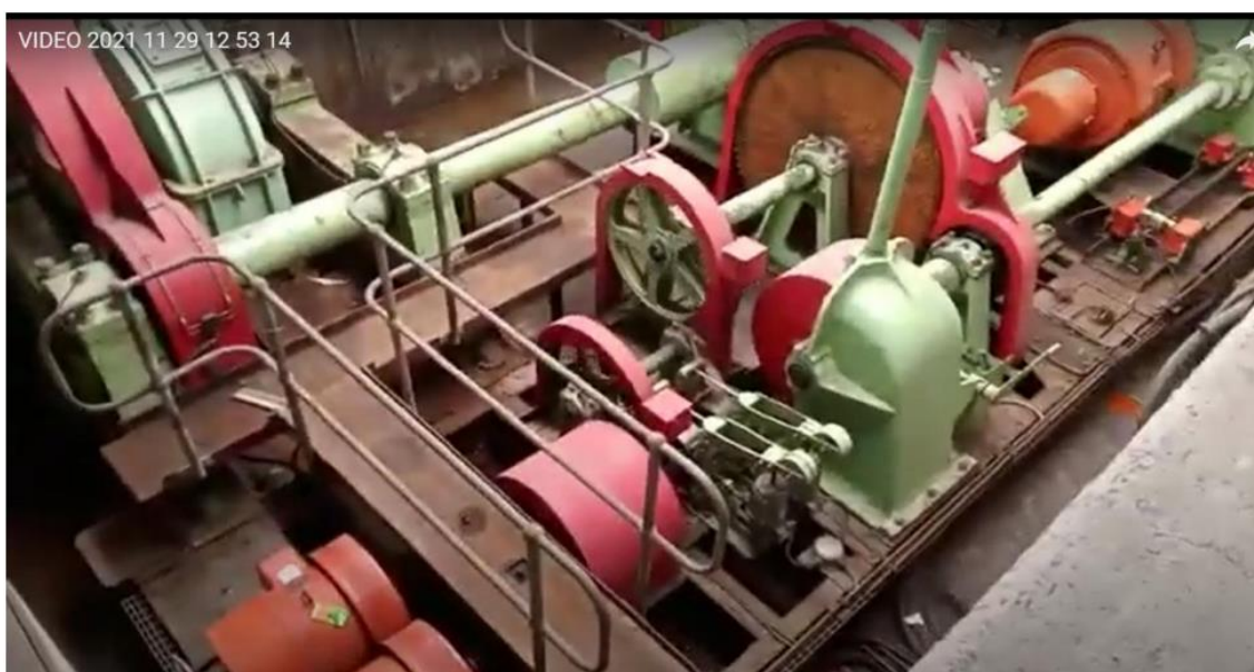
Figure 6 Winch House (Caisson Drive Train)
