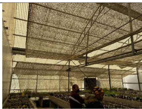
Picture 2: Existing manual pulley system hooks
