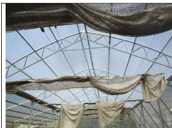
Picture 1: Existing manual pulley system
