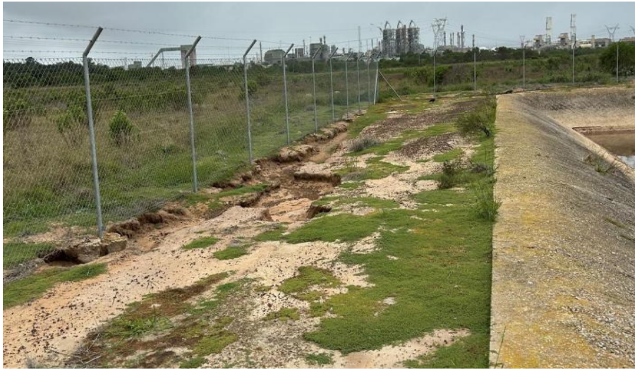
Figure 3: Typical Erosion Below the Fence
