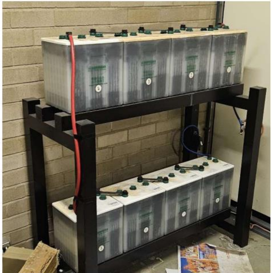
Batteries, Location: PABX Room Henley
