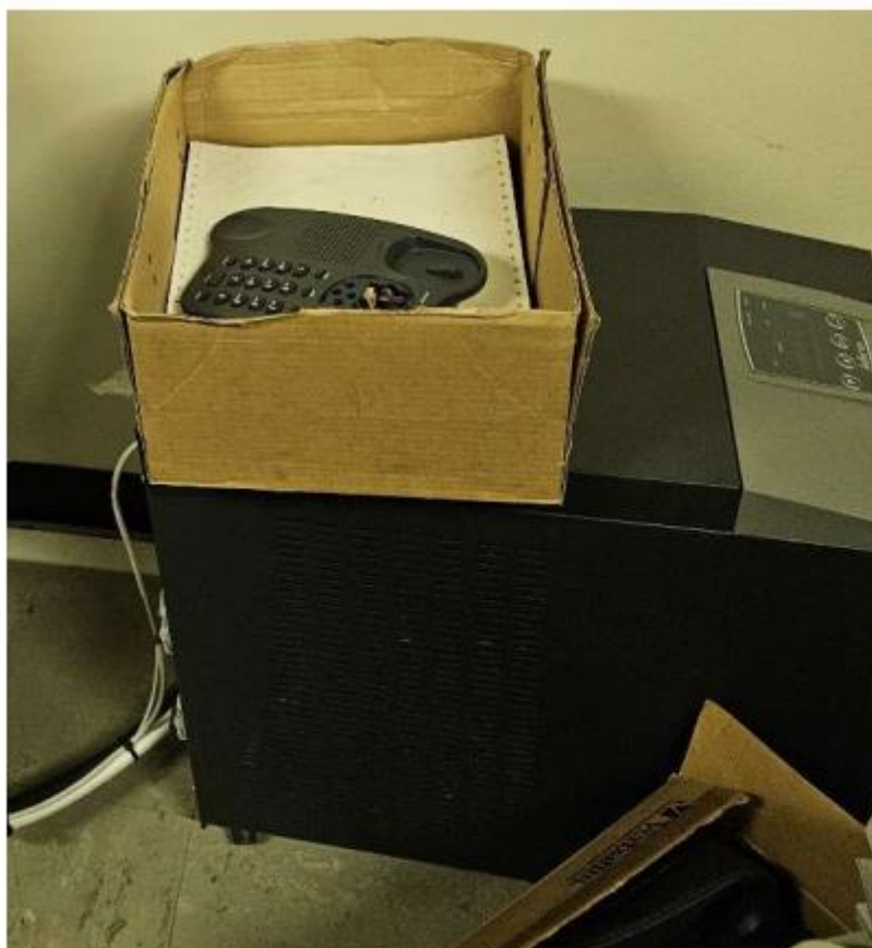
Battery Charger, Location: PABX Room Henley
