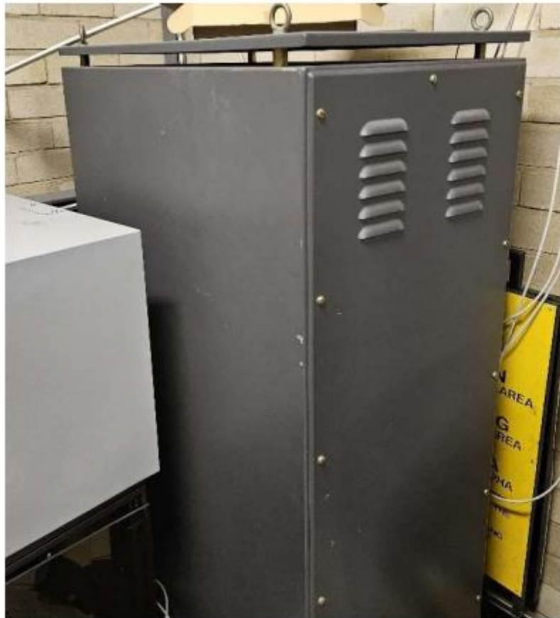
Battery Charger, Location: PABX Room Henley
