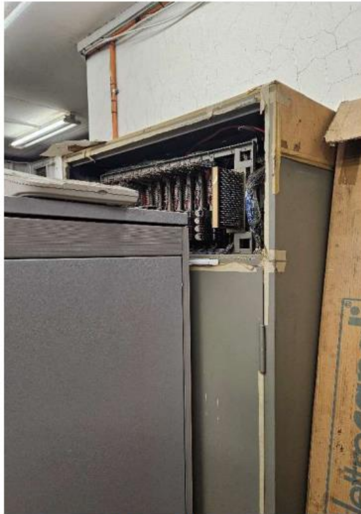
Telephone Philips PABX, Location: PABX Room K1
