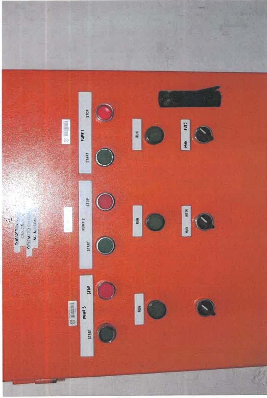
Figure 6: Existing Submersible Panel
