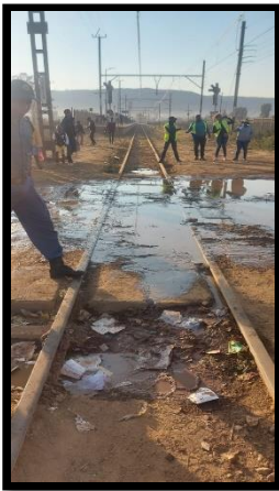
Picture 3: condition after rain events
