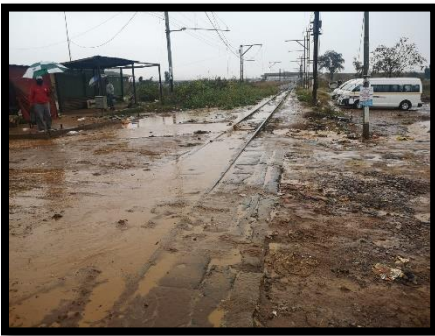
Picture 2: flooding during rain events
